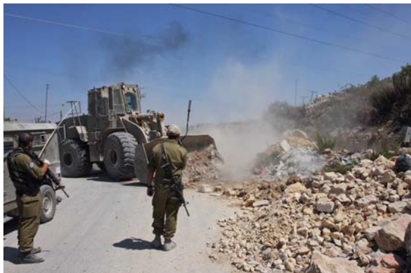
Israeli soldiers use a bulldozer to remove a roadblock at a checkpoint near Hebron.
